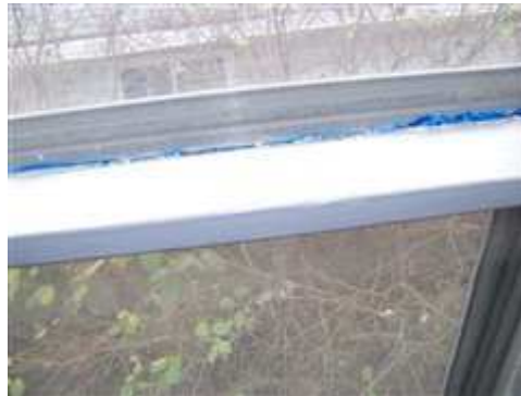
Photo 40 the lock is missing on this window
