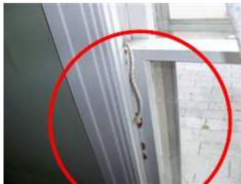
Photo 44 the rope s holding the counter weights has been cut.Window will not stay open without this being repaired
